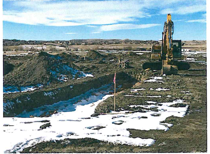
Village C Utilities
