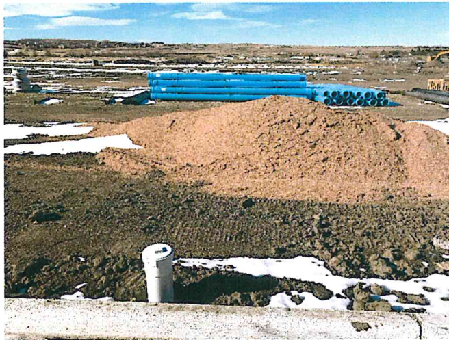
Underdrain along Interlocken Ave
