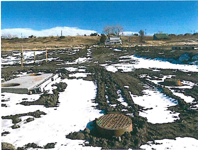
Village C Utilities
